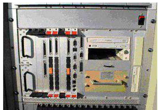
Signal Processing sub-rack
